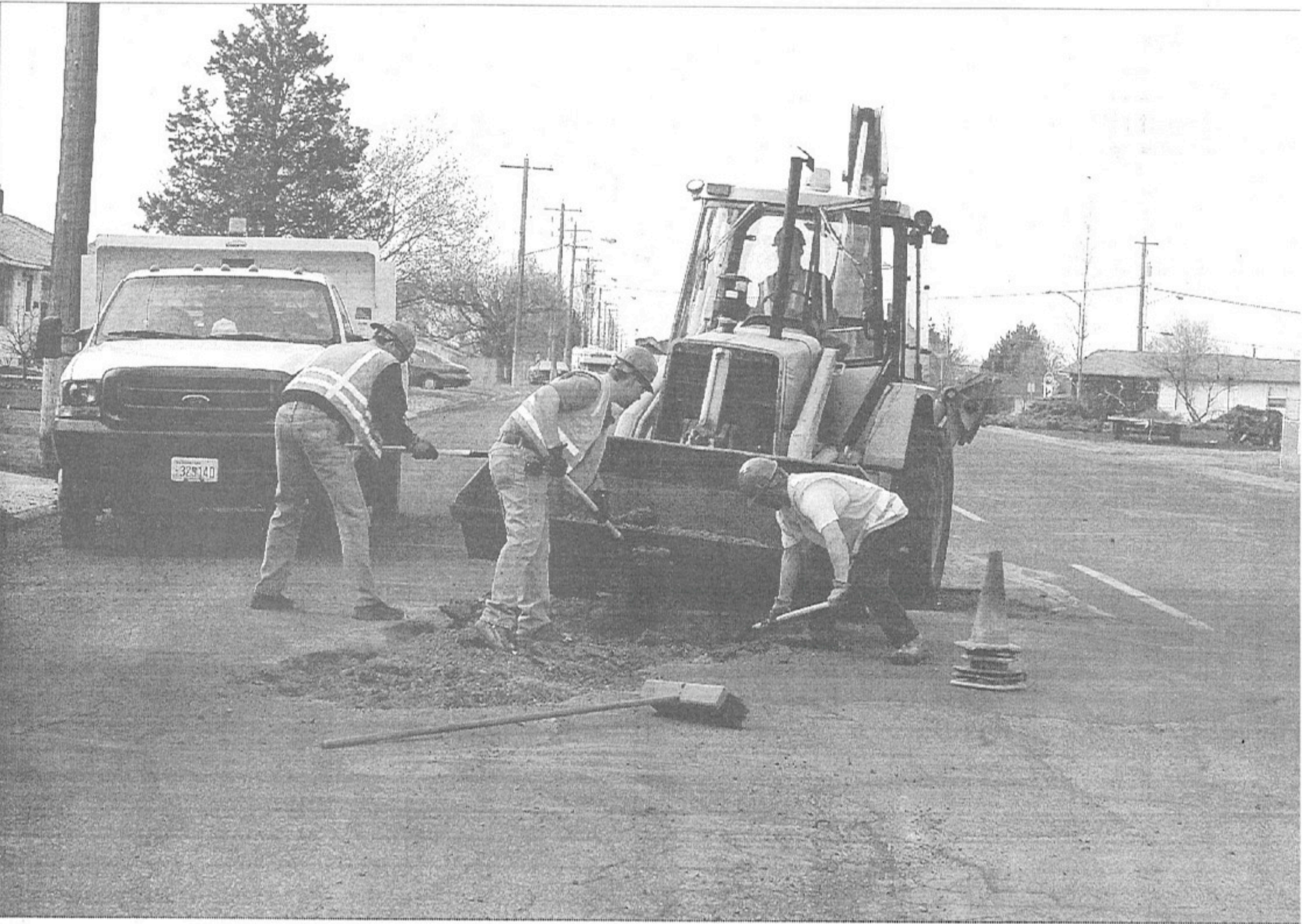
POTHOLE PATCHING SEASON UNDERWAY — An Ephrata Public Works Department crew cleans out a pothole on D Southeast Friday morning in preparation for patching. The city received its first batch of asphalt for the season this morning and work is now underway patching damaged streets throughout town after a winter that was particularly rough on residential streets. The city has scheduled an information open house on the proposed street and waterline repair and replacement project at 6:30 p.m. May 2 in the Ephrata City Hall.
